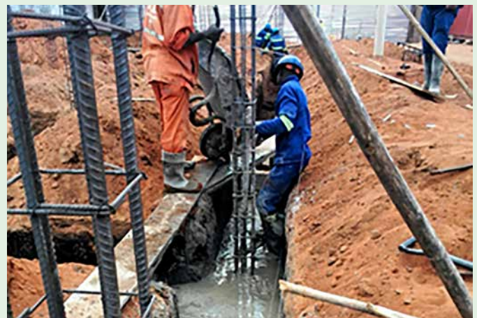
▲ The foundation was cast by hand by local workers. The iron rods and cables for the load-bearing columns are highly visible. SolidarMed
