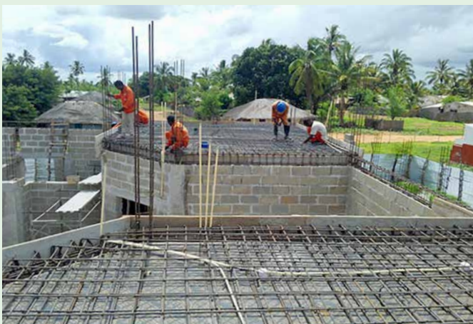
▲ At the turn of the year, the roof slab of the operating theatre was concreted and the electrical cables protected. SolidarMed
