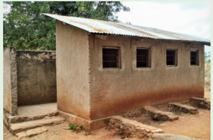
▲ The toilets in Ngoheranga Secondary School in Malinyi are finally being renovated in 2022. Benatus Sambili
